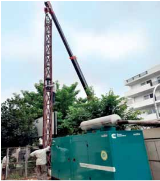
DG Installation with Stack for Exhaust Pipe at Sushant Lok-III Gurgaon
